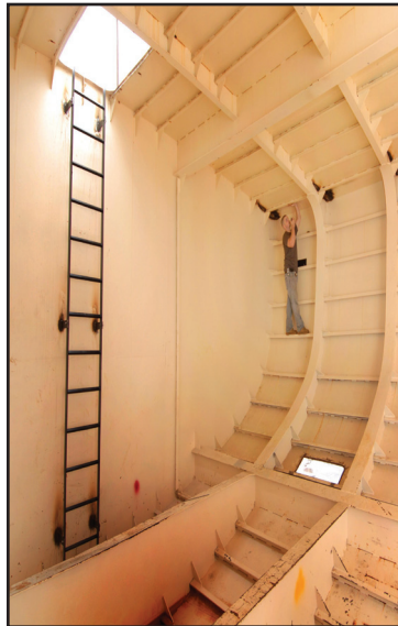
Benjamin Shulver of Ocean State Technical Services checks the quality of welds in the cavernous hull of the school ship Oliver Hazard Perry . photo courtesy of Larry Maglott
